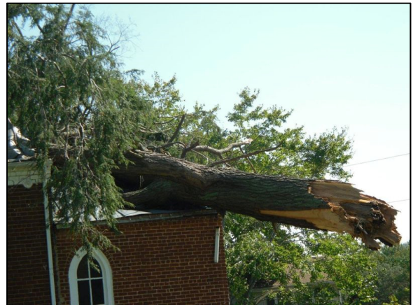
Figure 44- Christ Church (062-0003) was damaged by a September 2012 storm (photo courtesy: J.P. Harvey, nelsoncountylife.com)
