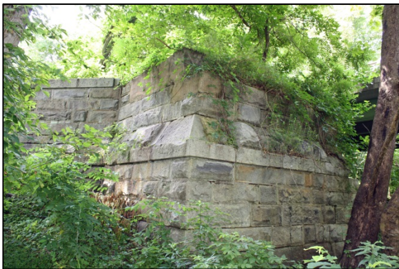
Figure 15- Finely crafted stone bridge abutment (ca. 1849) (062-0035) on the south end of the Route 56 bridge over the James River in Buckingham County.
